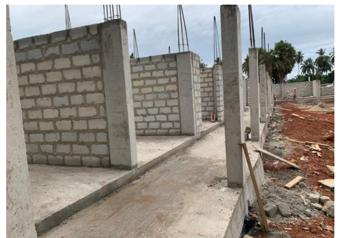
50 No. Lockable Stores, Paving of Market Area, Drainage Works, 1 No. Butcher Shop, 6 No. Open Sheds at Saltpond
