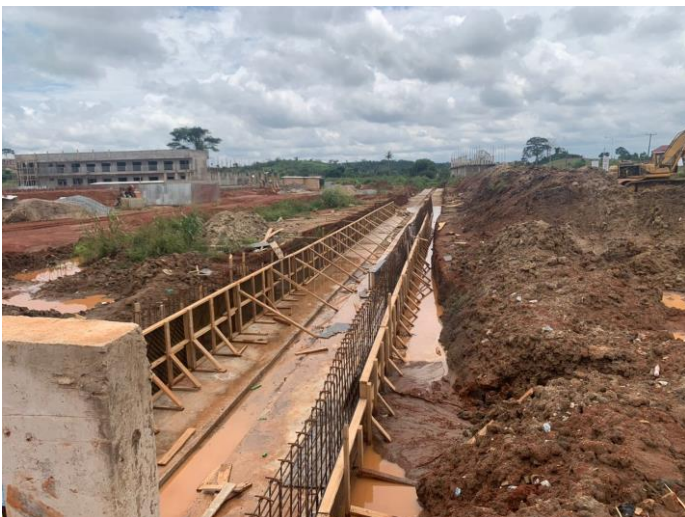
External Construction works at Mankessim (Site Preparation and Clearance, Access Road, Box Culvert, U-Drain, Electrical Installation and External Water Supply and Distribution)-UDD-3-Lot 2
